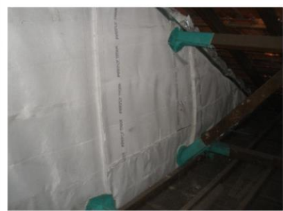
Roof Compartment Fire Barrier
