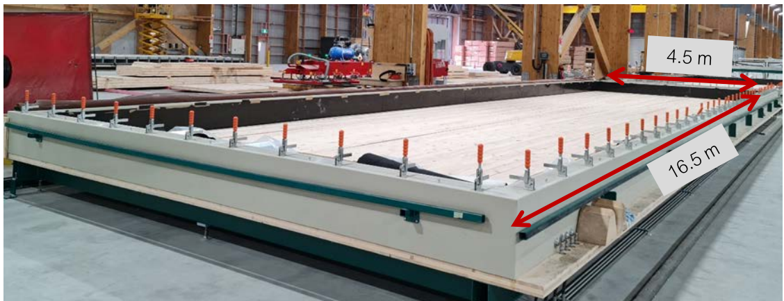
Figure 2: One of Red Stag's CLT vacuum presses.
