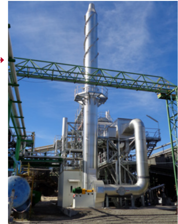
On-site energy centre →
