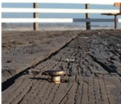
Spike pop-up hazard
