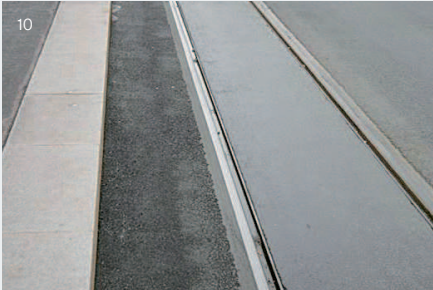
Step 4: The longitudinal joints between track and road are sealed permanently elastically (see picture 10).
